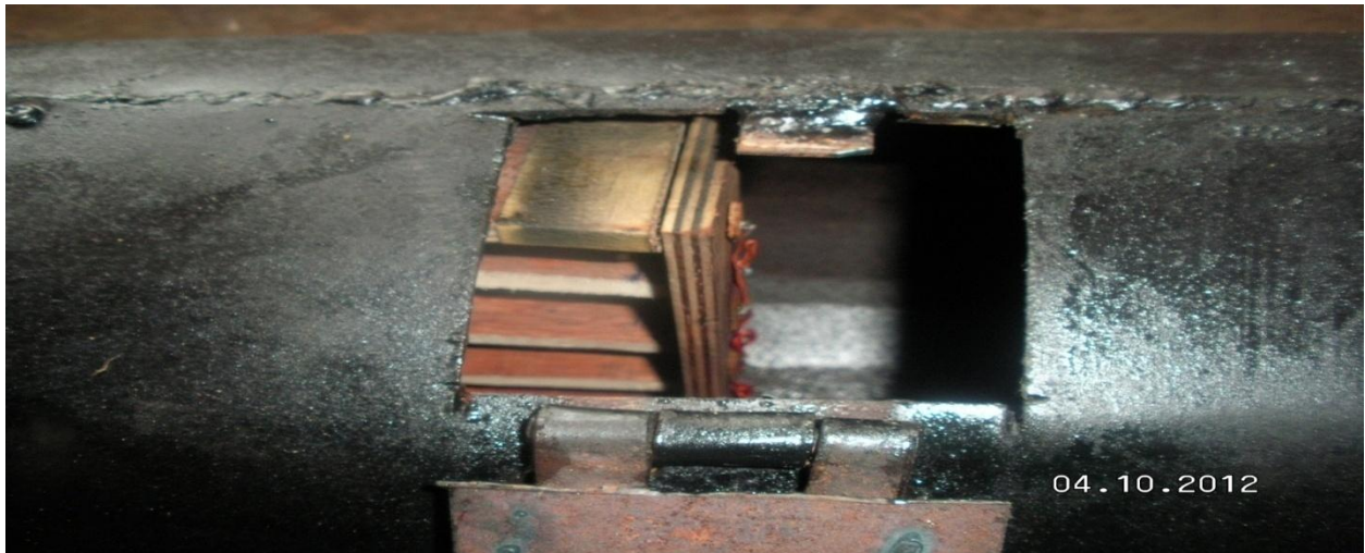
Fig 10: internal view of underground storage fuel tank and measuring system
